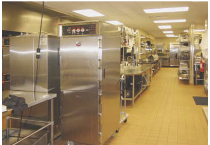
The large, fully equipped kitchen supports the R&D Catering Banquet facility and Ready Randy's Sports Bar & Grill.
