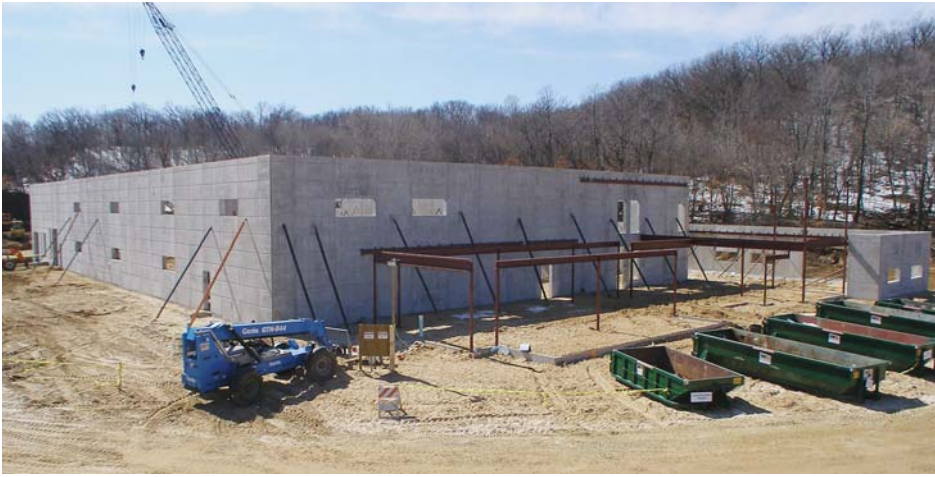
This photo of Air Motion Systems in River Falls, Wisconsin, was taken by our webcam in early spring, when the precast concrete panels and structural steel were being installed.
