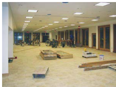
Pictured at left: St. Bridget's new fellowship hall just prior to completion.
